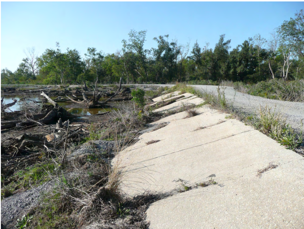
Figure 2: Segment of the pre-1926 levee still present in the Bohemia Spillway. The river (flood side) is on the left side of the levee/road. The elevation of the road bed on the levee is approximately 8 feet NAVD.
